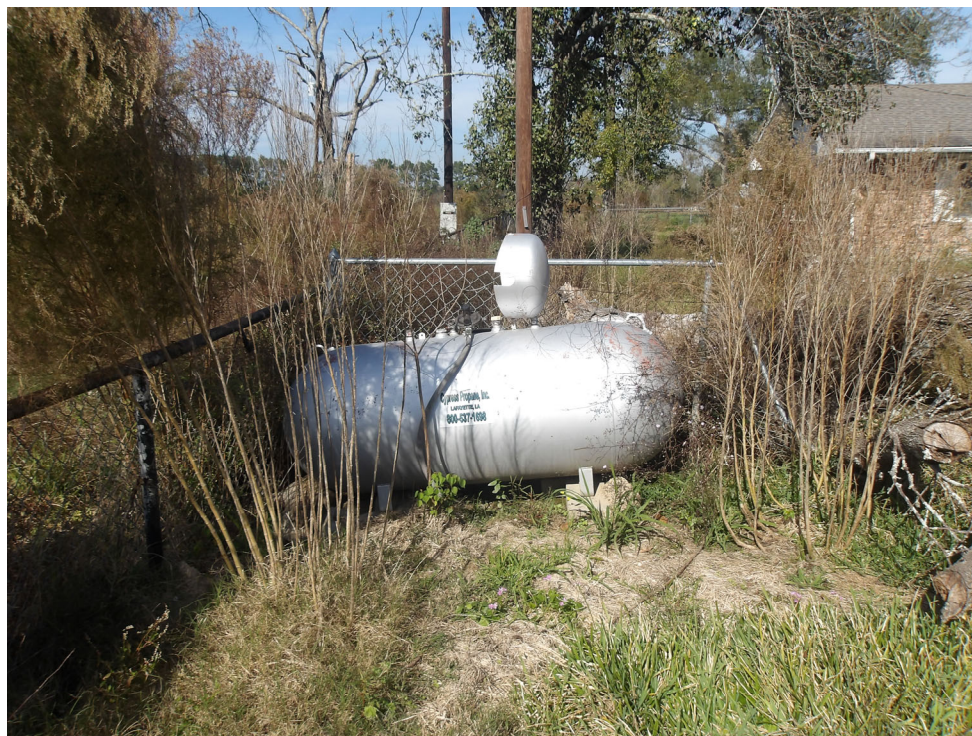
Photo 13: PL8 of propane tank facing north taken 11/26/2024
